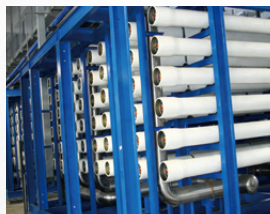
10000 tons/day Prince Paper Wastewater Phase II Retrofit Project
