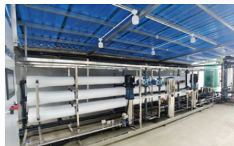
80000 tons/year Phosphorus-Containing Wastewater Compliance Discharge Demonstration Project
