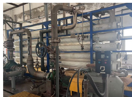
1000 tons/day Chlor-alkali Denitration Project – Nanofiltration Membrane Section
