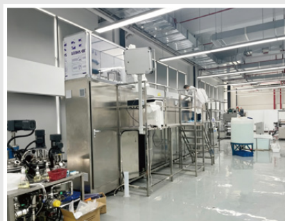
Hollow Fiber Membrane Production Line
