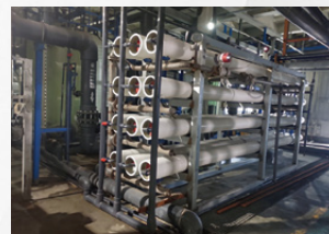
Annual output of 1,000 tons Lithium Carbonate Salt Lake Lithium Extraction Demonstration Project
